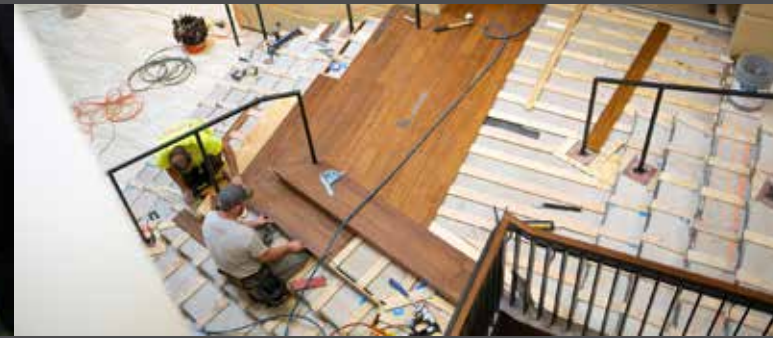
1 MILLION-PLUS Feet of wire used throughout the building
