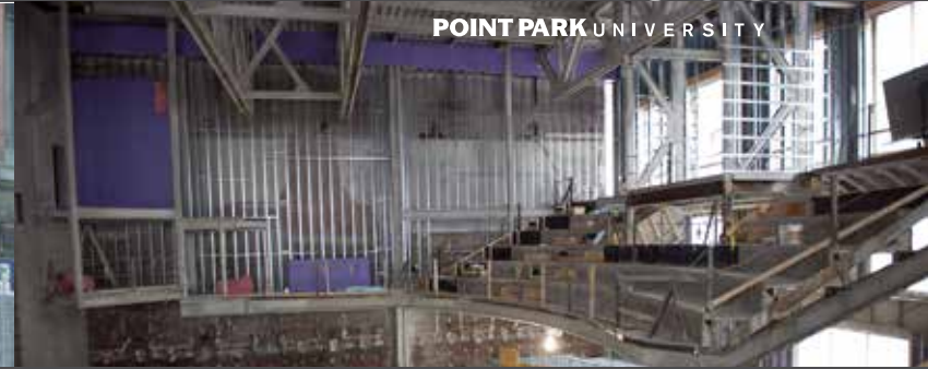
30,000 Feet of galvanized aircraft cable used for stage rigging
