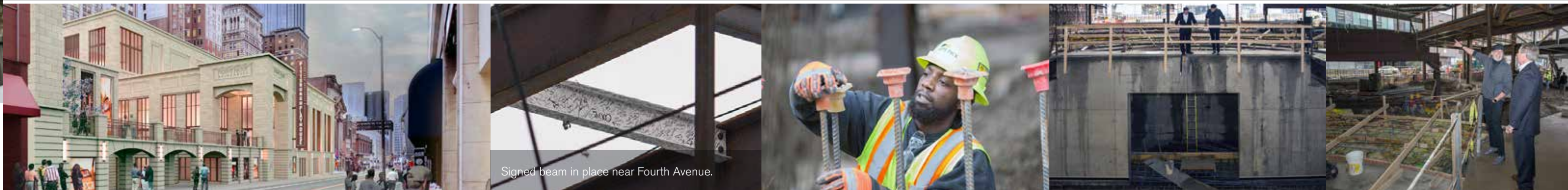
Point Park President Paul Hennigan and Conservatory of Performing Arts Artistic Director Ronald Allan-Lindblom survey Playhouse construction. Photos by John Altdorfer.
